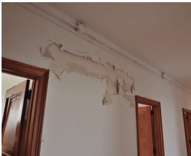
Figure 80. Infiltration toit, BGLA
