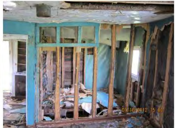
Image 29-HaGa-1, House: View of vents along south wall in dining room.
