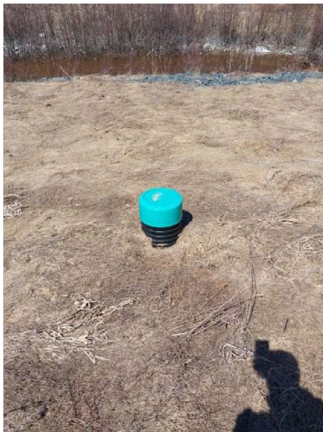
Photo no. 9. Boite de service est.
