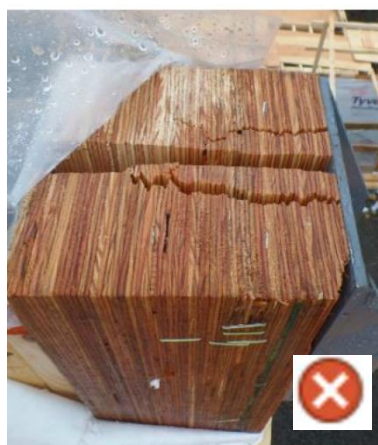
Photo 6 – fissuration (pré-perçage non conforme
