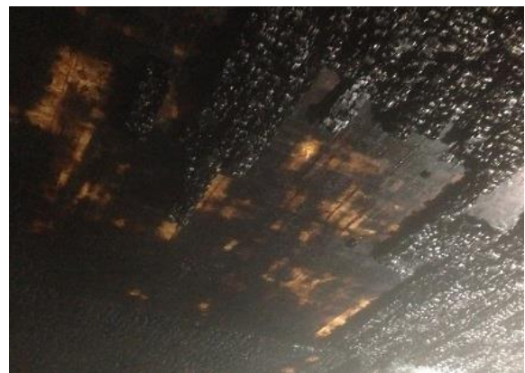
f) Ceiling assembly showing localized delamination
