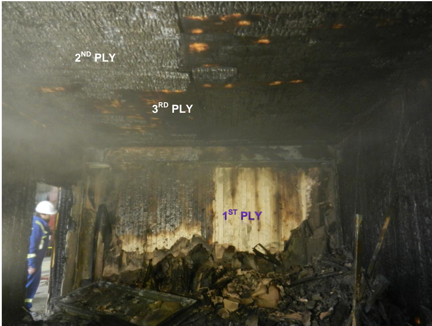
Figure 32. Inside of the fire compartment after the fire demonstration.
